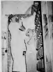
Adolph Arends cuts hundreds of temporary jumper wires that kept the two exchanges linked, while Carlino Henriquez cuts hundreds of old exchange incoming wires.
